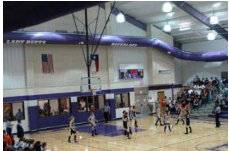
Figure 10.9 DuctSox Florence, Texas gymnasium with customized fabric ductwork
